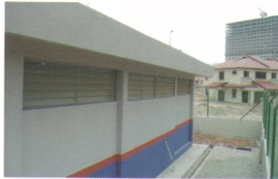
Substation Window Panel
